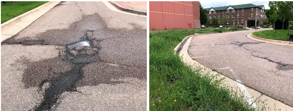
Figure 2. Poor Provision of Street Improvements
