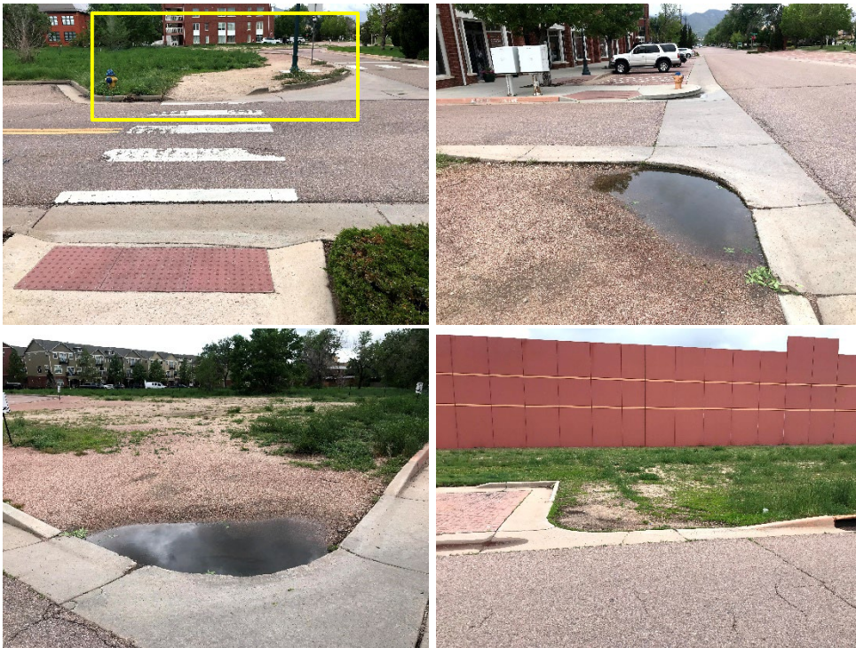
Figure 3. Lack of Sidewalks
